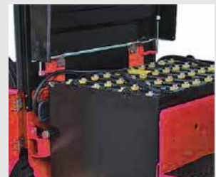
The battery cover can be fully opened, the design is easy for maintenance
